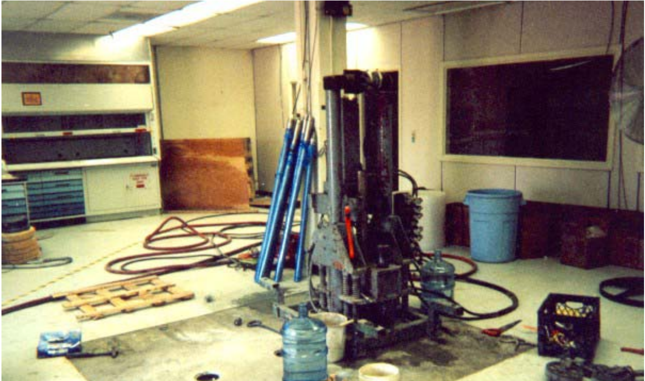
Figure 4-5. Indoor Vibra-Push Rig (LD Geoprobe® Series) Used in the Engineering Support Building
