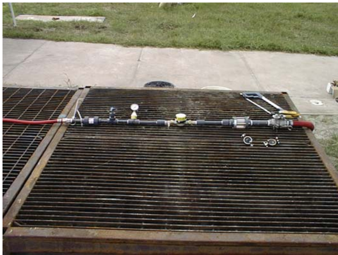
Figure 3-4. Oxidant Preinjection Manifold
