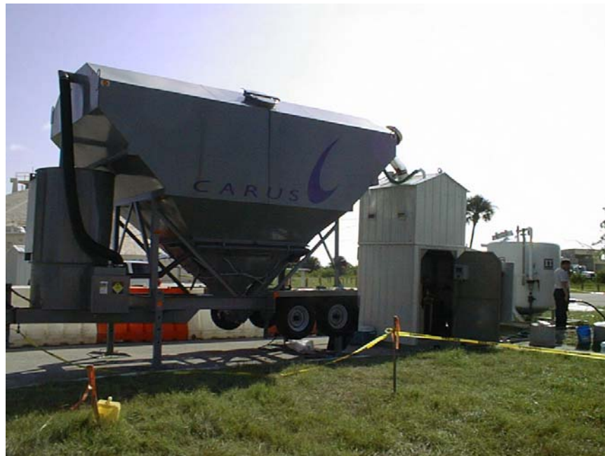
Figure 3-3. ISCO Setup at Launch Complex 34 Showing Permanganate Storage Hopper and Mixer
