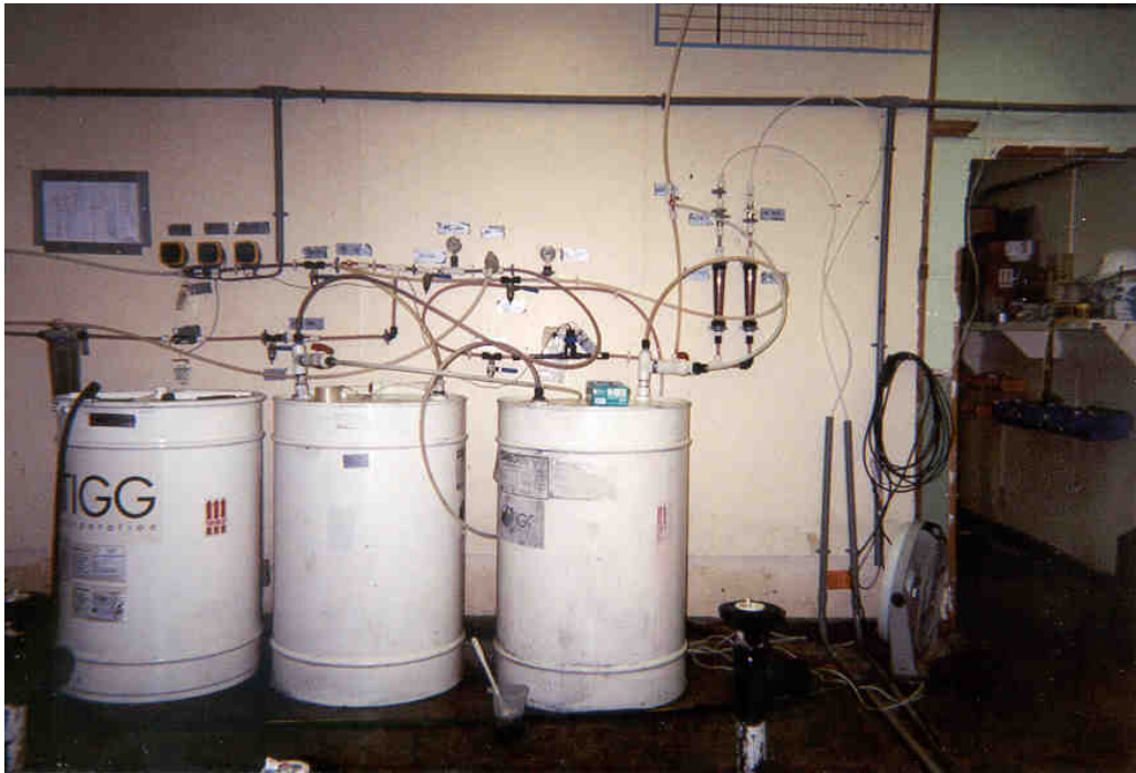
Figure 3-4. Aboveground Water Treatment System (A Series of Two Carbon Tanks and a Backup Tank)
