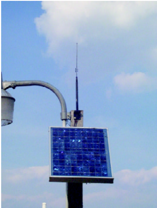
Figure 4.3 Solar Panel (Stonington Site).
