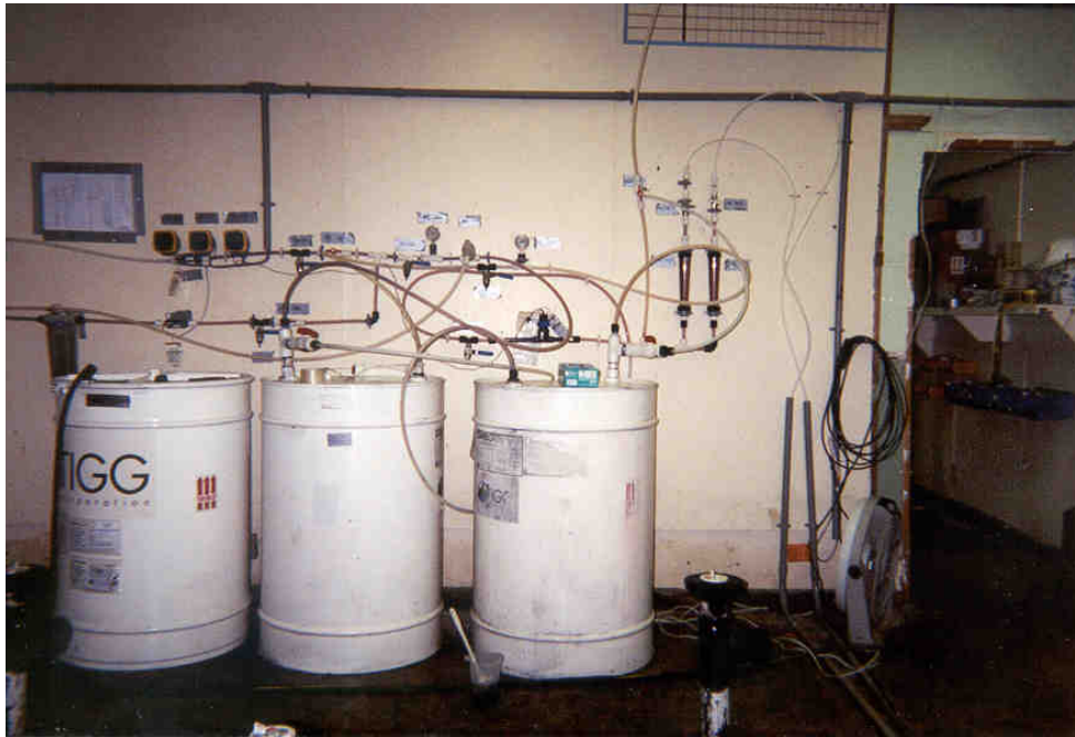
Figure 3-1. Aboveground Water Treatment System
