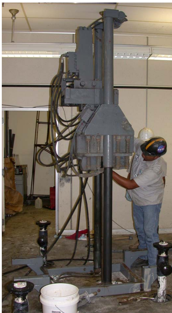
Figure 4-5. Indoor Vibra-Push™ Rig (LD Geoprobe® Series) Used in the Bioaugmentation Plot Inside the Engineering Support Building
