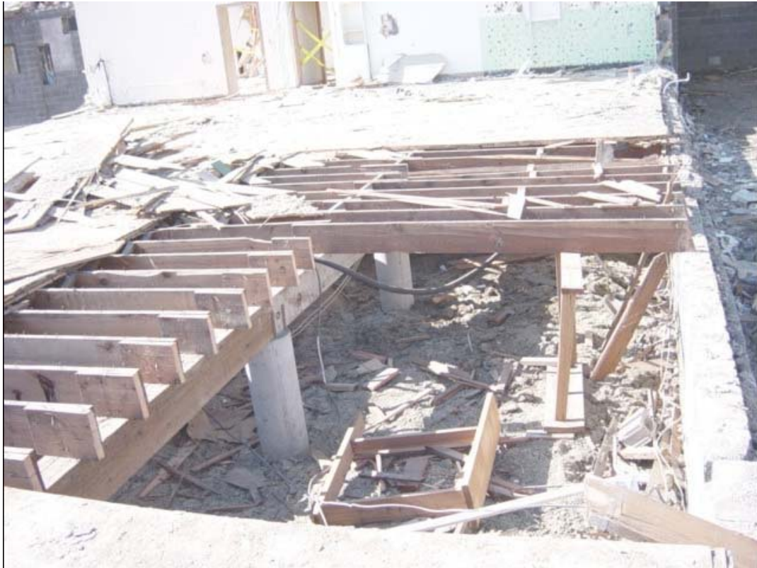
Figure A13. Floor joists and concrete piers exposed during deconstruction of building 6286.
