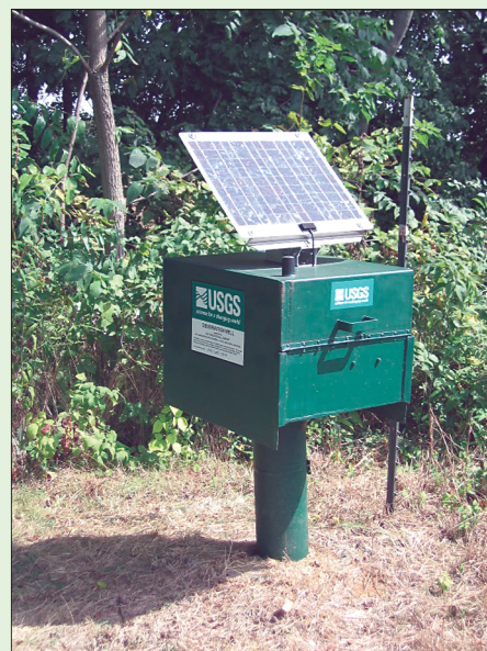
Observation well WA Ci 82 in Washington County, Maryland, with near-real-time transmission equipment. (Photograph by Charles J. Strain, USGS)
