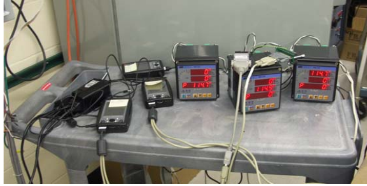
Figure 16. SCMs and Meters Used for DNP Demonstration at DTE Energy
