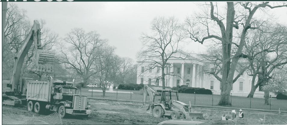
Construction crews pave the way for the redesign of Pennsylvania Avenue at the White House.
