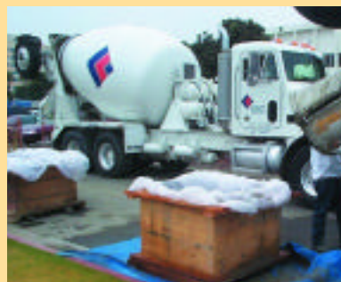
<Wastes from concrete truck stored in wooden box to prevent runoff of construction wastes into the street and the bay>
