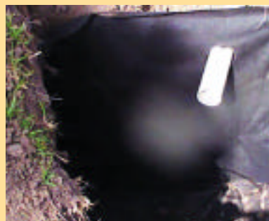
<Sub-surface drywell with filter fabric lining and 2 influent pipes from roof>
