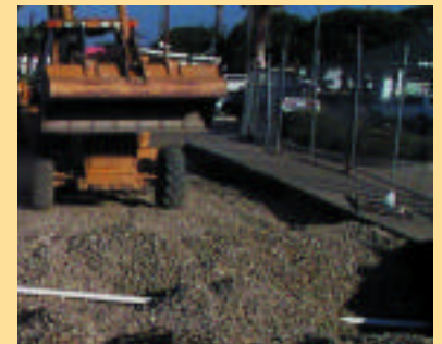
<Runoff from supermarket parking lot is diverted into this large drywell system, which is under the parking lot>
