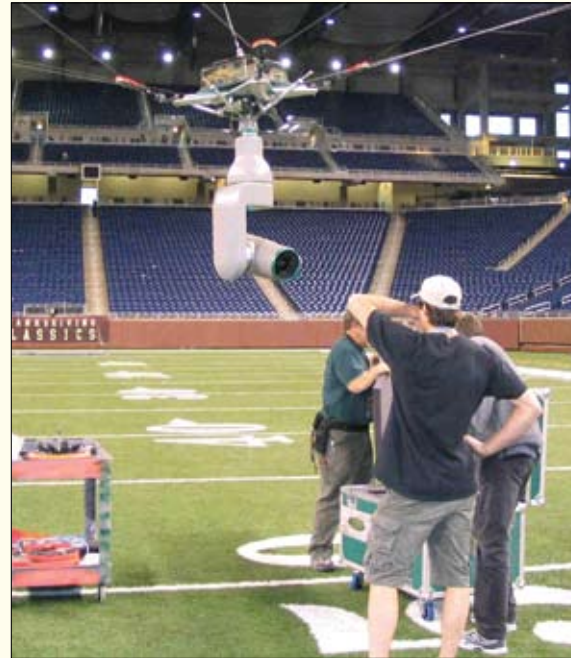
System installation of the gimbal technology at Detroit's Ford Field, Thanksgiving Day 2004.
