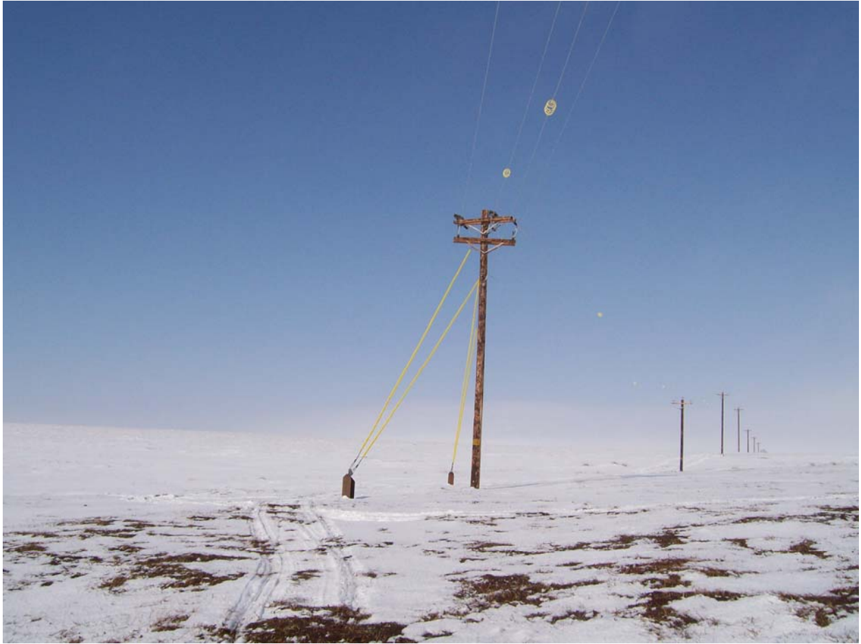
Toksook Bay to Nightmute 13.8kV intertie. Photo courtesy of Alaska Village Electric Cooperative.
