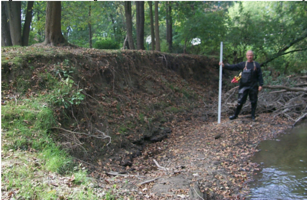
Figure 5.1: Mass Wasting and Bank Failure located at Reach 13 in the Pilot Study Site
