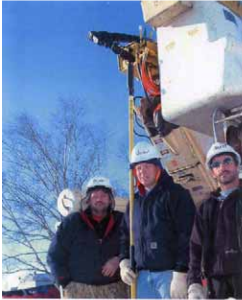
Figure 1. PCB transformer phase-out (Grand Marais, MN).
