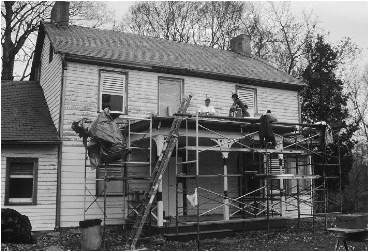
Park construction crew led by preservation carpenter Doug Townsend rehabilitates the covered porch. A new flat seam metal roof was installed with assistance from the NPS Historic Preservation Training Center in Frederick, MD. NPS photo.
