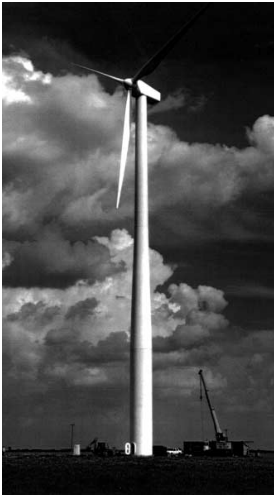
THIS WIND TURBINE near Clovis, N.M., and another (site to be determined) are expected to provide electricity for approximately six percent of the DOE's Waste Isolation Pilot Plant (WIPP) total electric services requirement.
