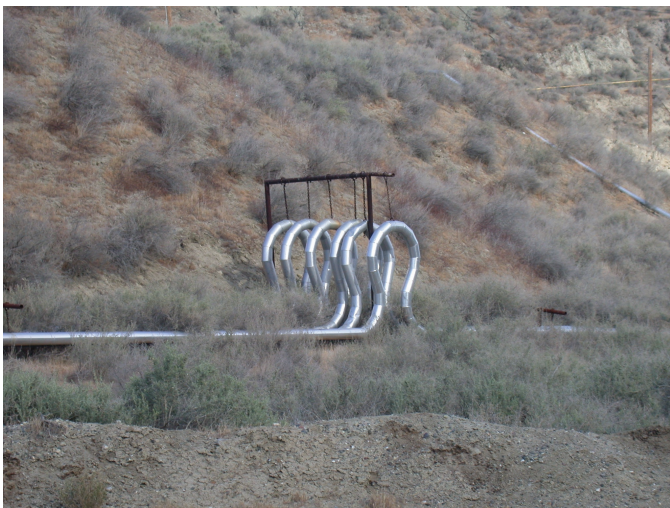
Figure 3.58. Steam lines and other equipment associated with steam technology take up space in this oil field near Coalinga in areas once used to feed and house oil-field workers and their families.
