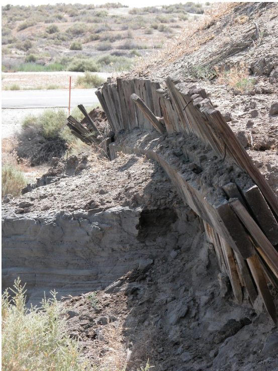
Figure 3.38. Wooden structure that was part of a dike built to contain the oil from Lakeview 1.
