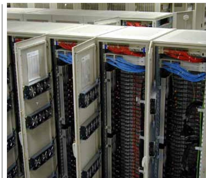
Interior of the Sandia-built C Plant parallel computer, showing its many racks of processors
