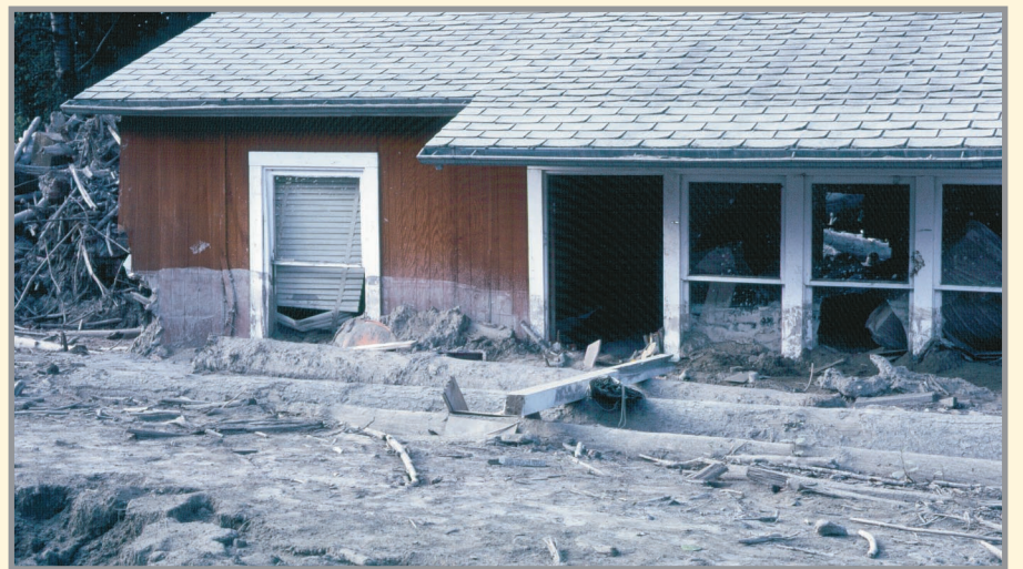
House partly buried by lahars from the 1980 eruption of Mount St. Helens. Note the high mud line on the house and large amounts of woody debris carried by the lahars. (Photo by Lyn Topinka, USGS)
