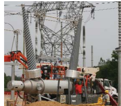
Substation Expansion Erial, NJ
