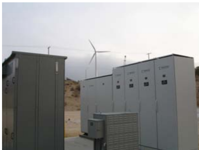
EnergyBridge System Installed at Palmdale (May 2008)
