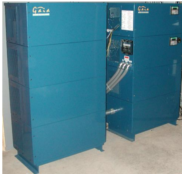
Figure 2. PowerTower and Main Communications Panel
