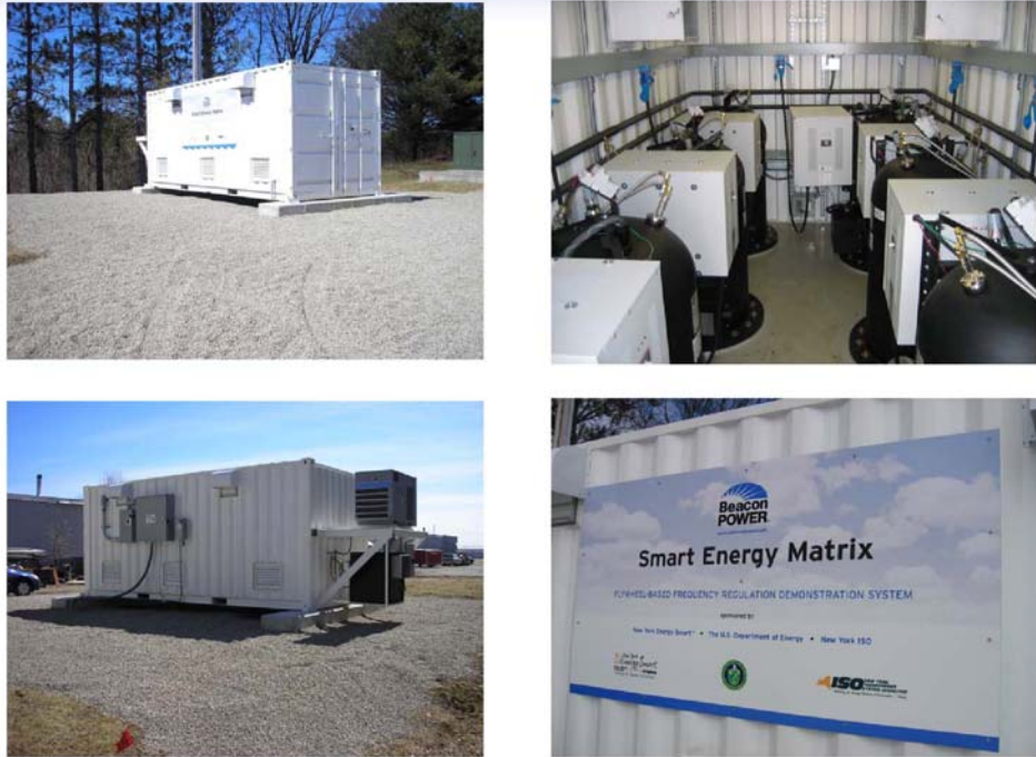
Figure 9. The Beacon Smart Energy Matrix FESS Installed at the PCT Site
