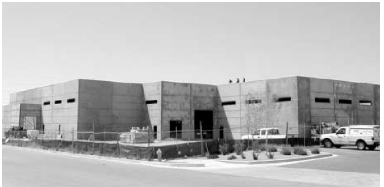
NEW NEIGHBOR — Ktech Corp.'s new 80,000 sq. ft. facility is under construction at the corner of Eubank and Gibson SE in the Sandia Science and Technology Park. Ktech, a strategic Sandia supplier, joins 14 other tenants that have chosen to call SSTP home over the past five years. Ktech plans to occupy the new facility in November.
