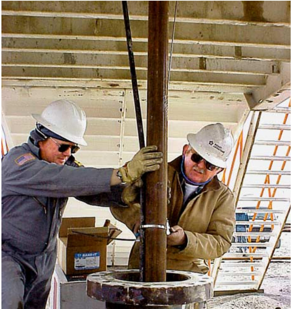
NEW TECHNIQUE — Jim Westmoreland, left, and Ron Jacobsen strap hoses to drill pipe at the Rye Patch well in Nevada to direct polyurethane grout into the well. The two members of Sandia's Geothermal Research Dept. 6211 were instrumental in proving that the new technique, using polyurethane grout, will work.
