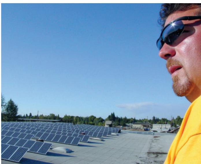
Figure 7: A bright future for solar energy This installation of photovoltaic (PV) panels in Eugene is just one example of the use of solar electricity.
