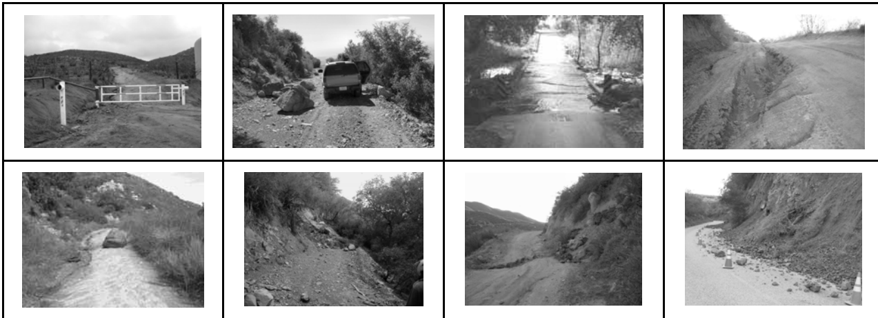
Rockslides, overflowing crossings, road closures, and road damage after the heavy and frequent rains early 2005, Cleveland NF
