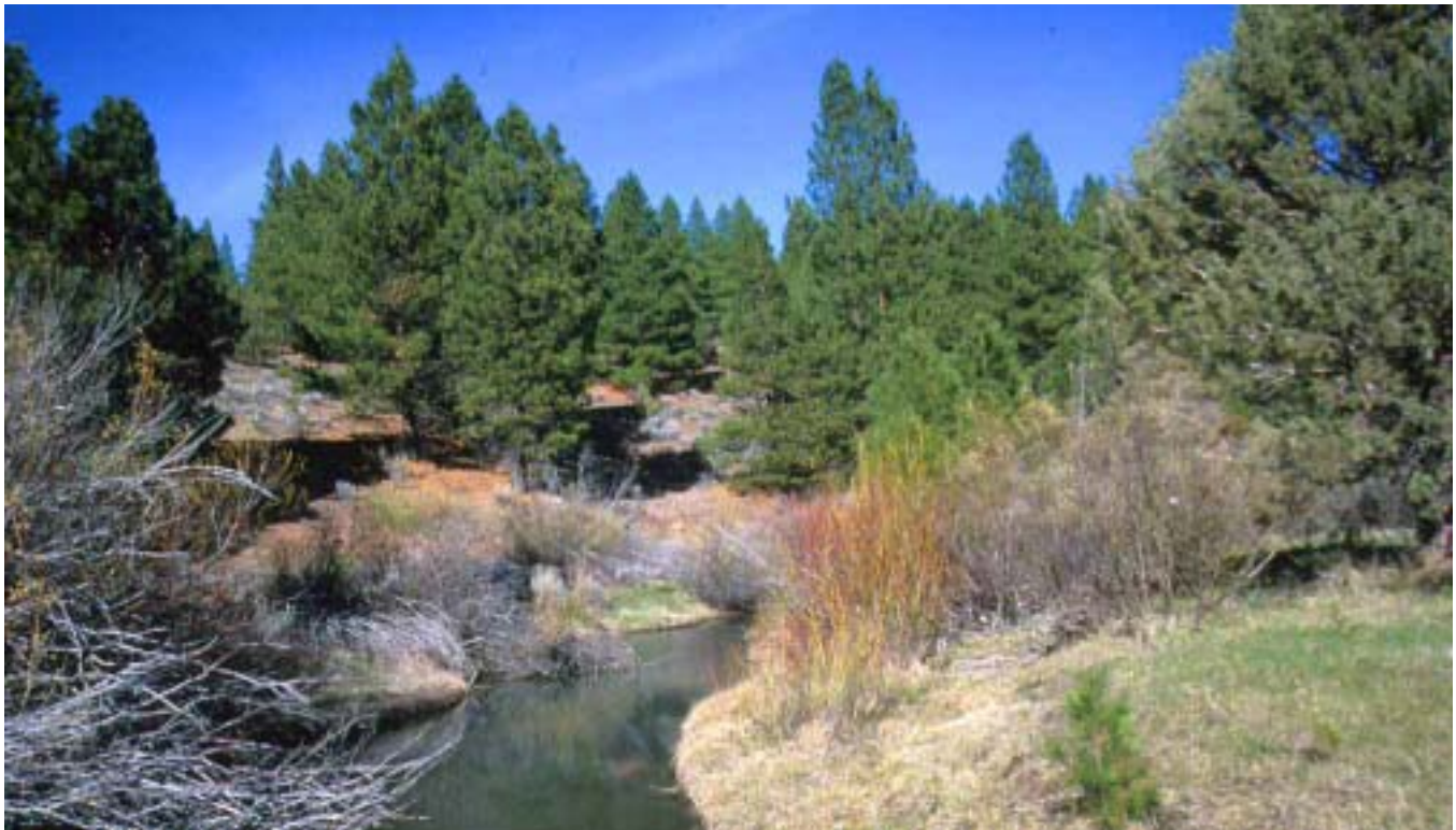
Lassen Creek Streambank Stabilization Project on the Modoc National Forest in Susanville, CA
