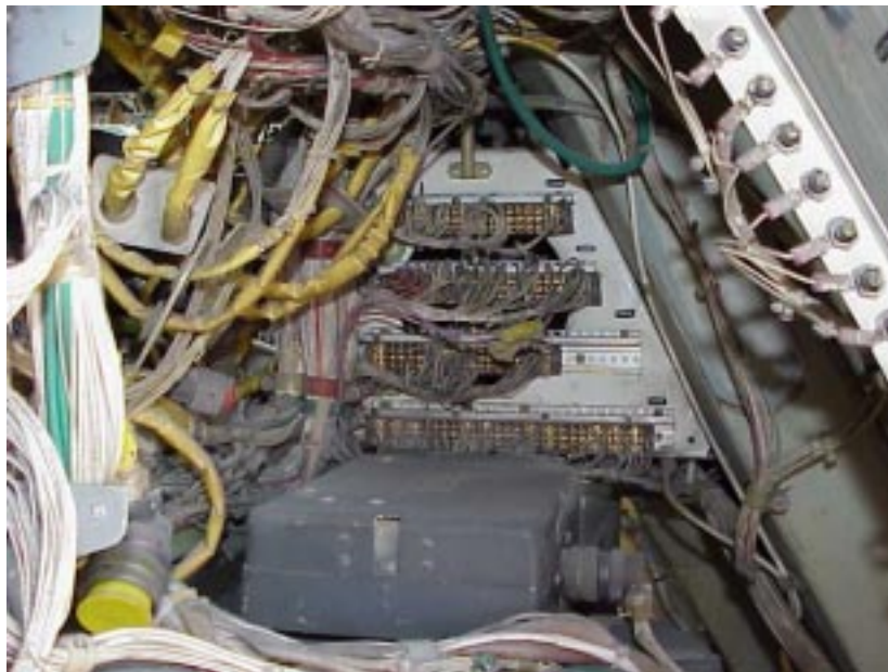
Figure 11. Typical installation of wire systems in a transport airplane.
