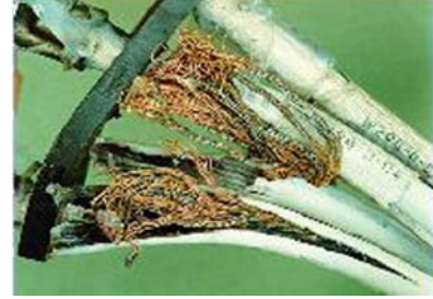
Figure 3. Wire failure mechanisms: thermal.
