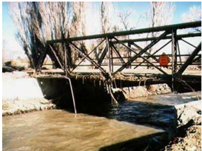
Figure 3 High water deposits debris and sediment on bridges and can damage their foundations
