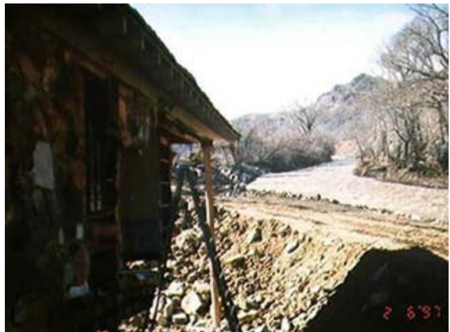
Figure 2 A constricted river channel caused the raging flood water to find a new path, carving a gorge under this house
