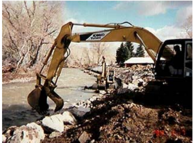
Figure 1 Immediate work to restore river channels protects private property from further flood damage
