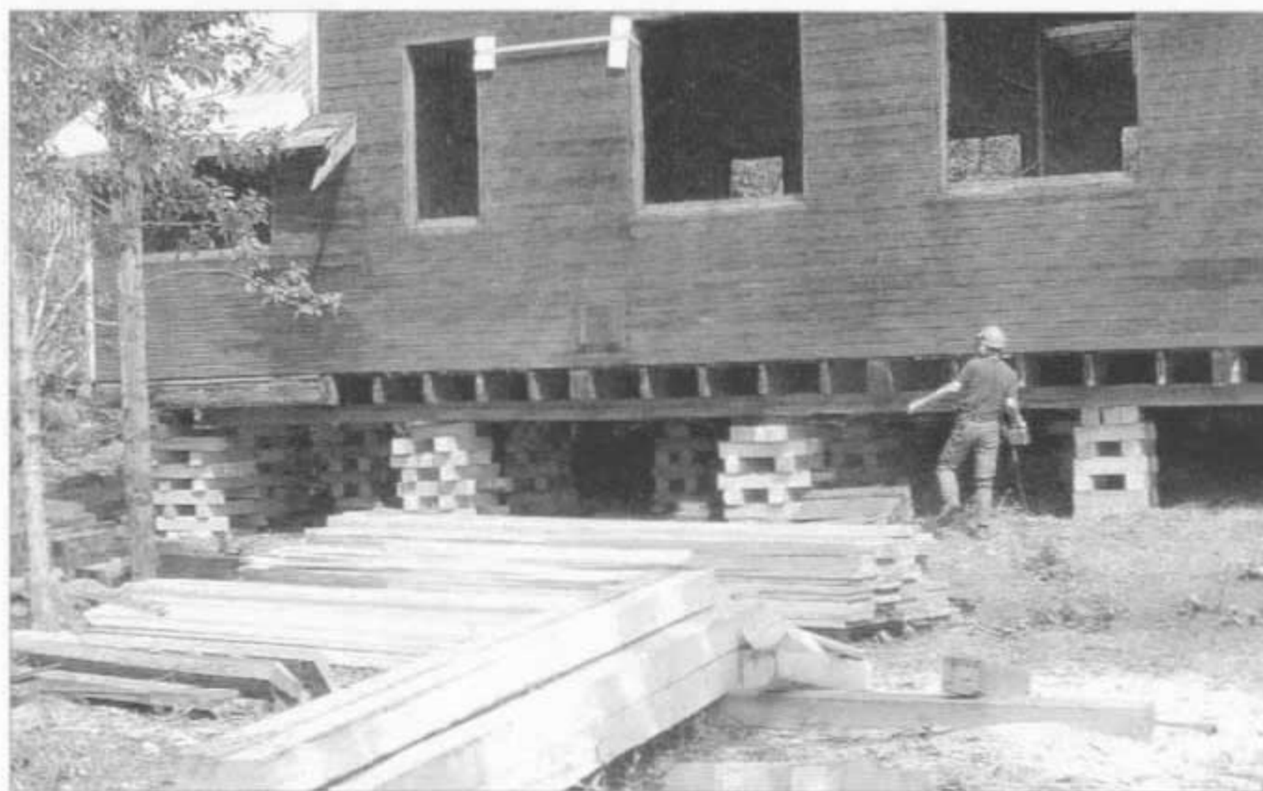
Park staff replaced the cribbing under the Kennecott Recreation Hall in 2001
