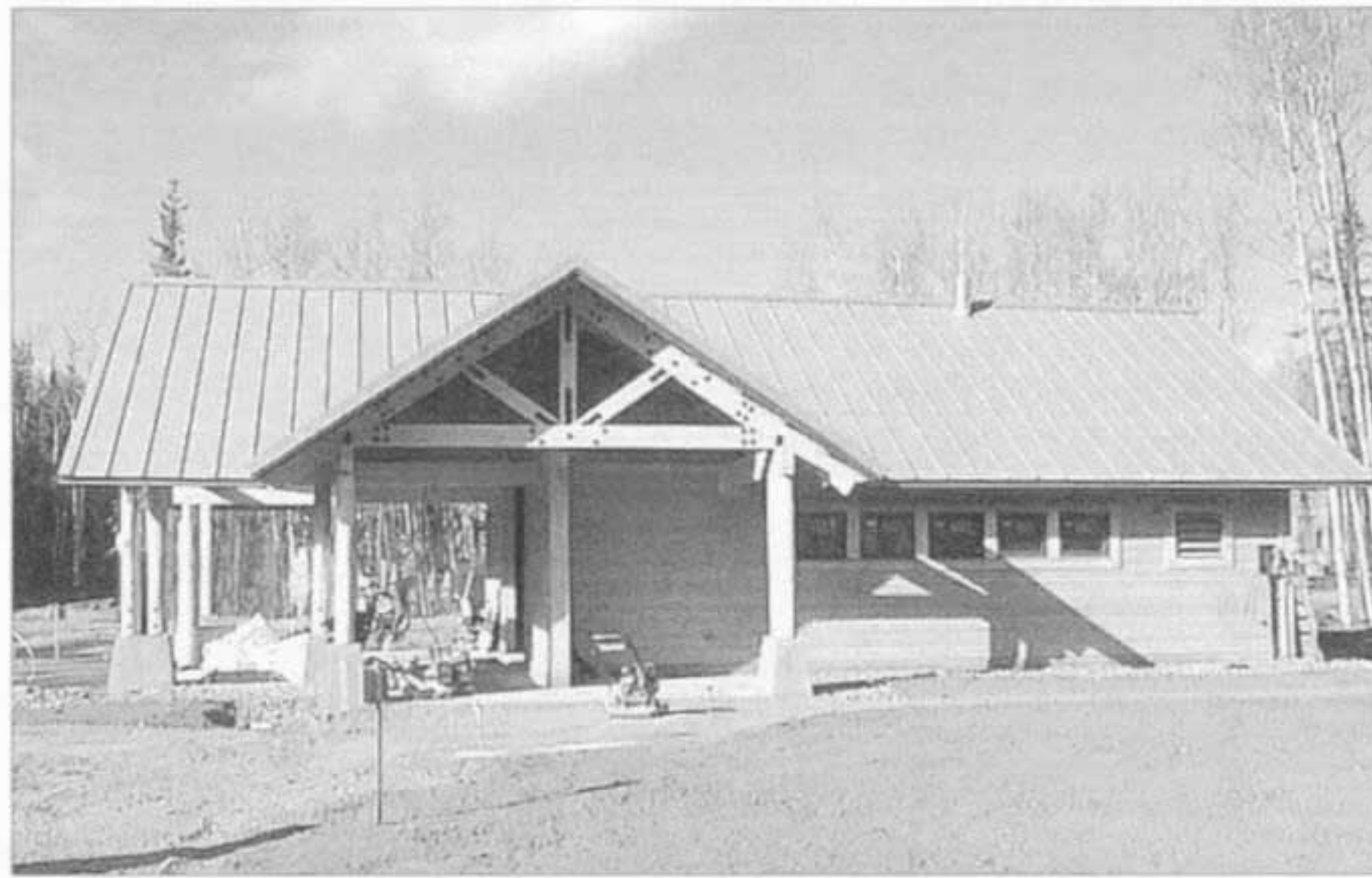
Construction of WRST's new Visitor Center is expected to be completed in early 2002
