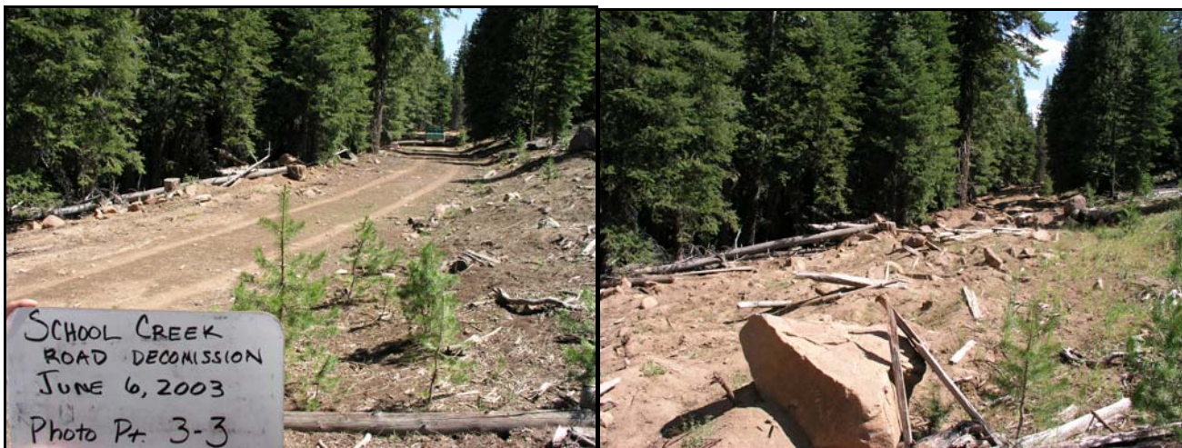
School Cr Road Decommissioning Paisley Ranger District Road Maintenance and Decommissioning project
