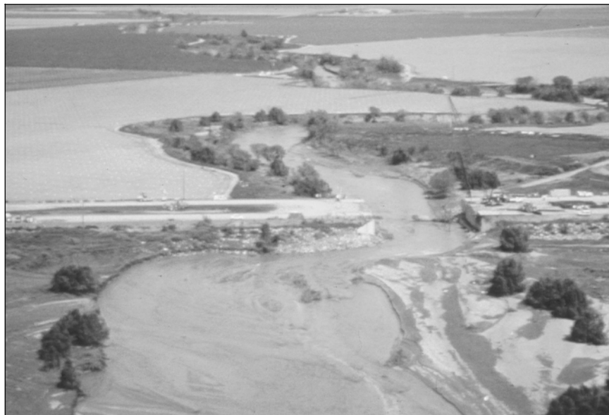
Figure 2.2. Live-bed contraction scour contributed to failure of the I-5 bridges near Coalinga, CA.
