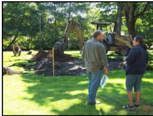
Breaking Ground - Above: MJ Kesterson (right) talks with contractor Rob Chisholm on the first day of groundbreaking for the new memorial. At left: A geologist prepares to take samples while surveying the digging site.
