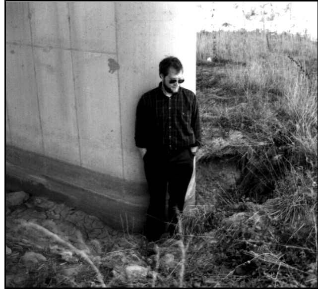
Figure 4-3. Local scour at a round-nosed bridge pier. Note protective vegetative cover of surrounding floodplain.
