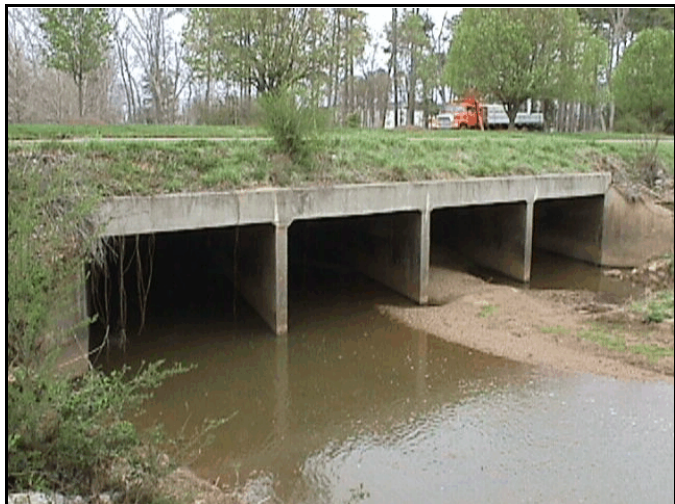
Figure 3-7. Bridges and culverts can be modeled well by one-dimensional flow approximations when their widths are small in comparison to the channel and floodplain.
