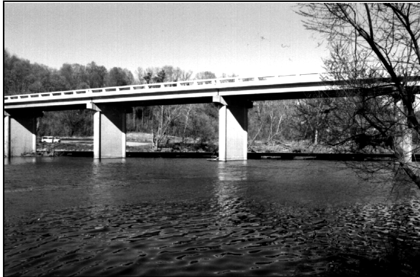
Figure 3-5. View of a bridge where two-dimensional flow would likely be modeled because of the comparatively large width of the opening.
