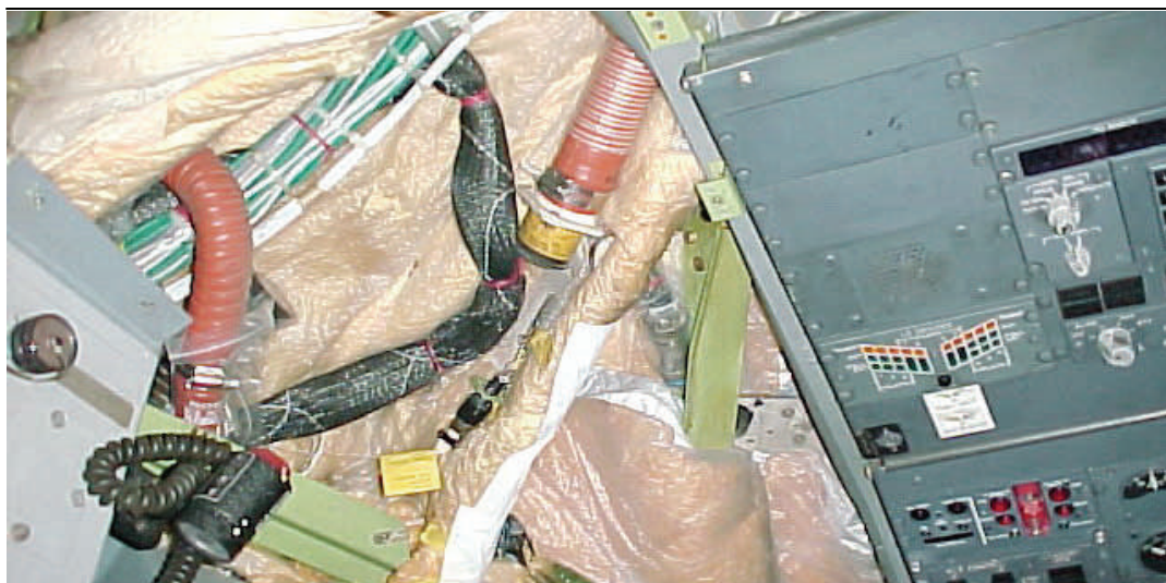
AN-26 around system wiring overhead in a flight deck is complex to identify and remove.
