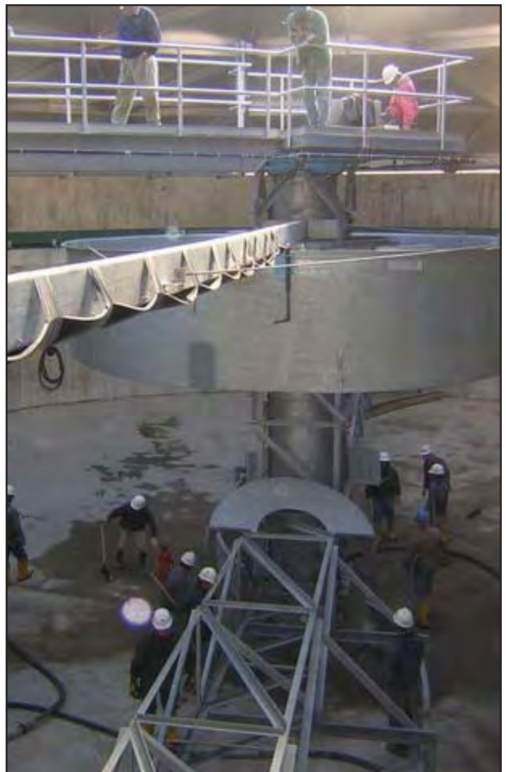
POTW Finished Clarifier in Sanford, ME.
