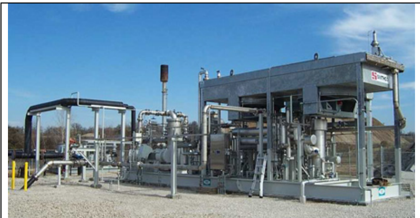
Figure 27 LFGE treatment/blower/flare station. Image courtesy LMOP 134
