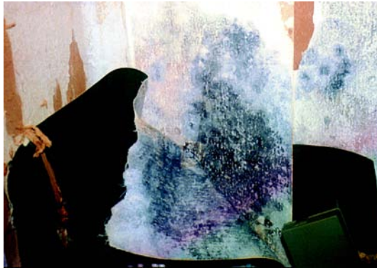
Photo 5: Mold growth behind wallpaper
