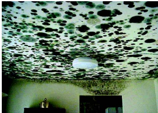
Photo 2: Extensive mold contamination of ceiling and walls
