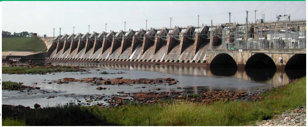
Progress Energy's Tillery dam and power plant on the Pee Dee River
