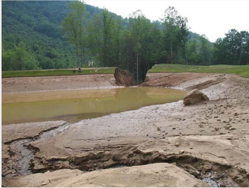
The compromised dam at Balsam Mountain Preserve
