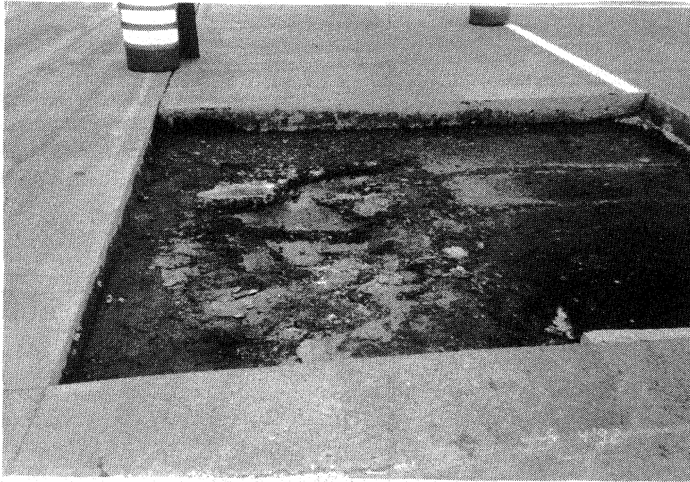
Figure 10. Erosion of subbase under punchout distress.
