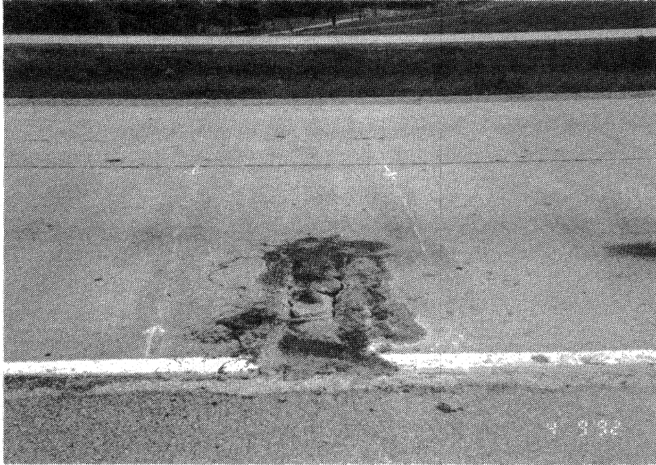
Figure 20. Marked out distress area.
