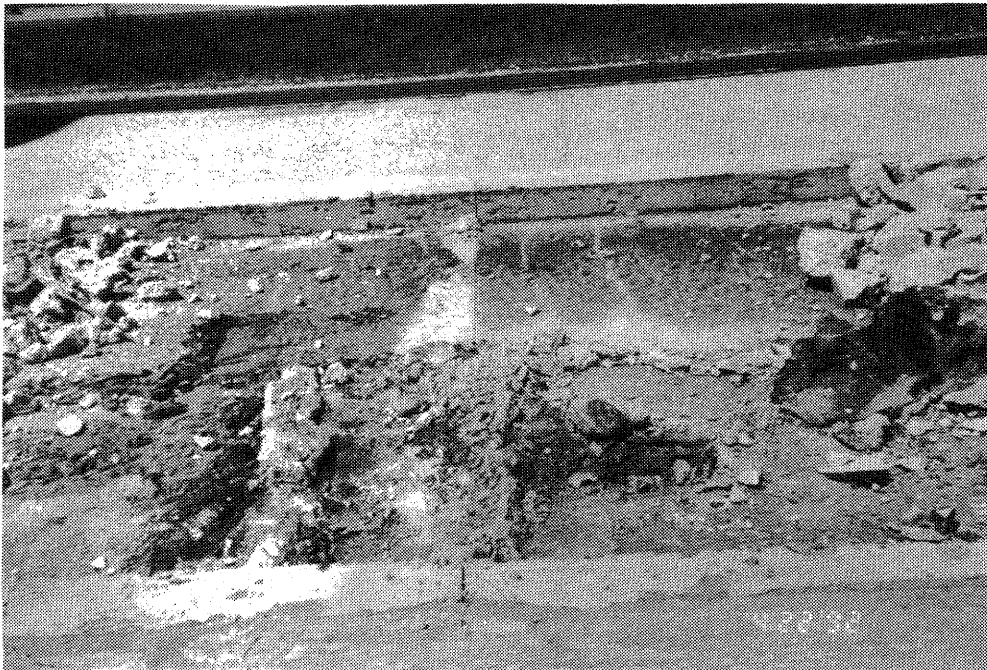
Figure 11. Movement of material caused by pumping.
