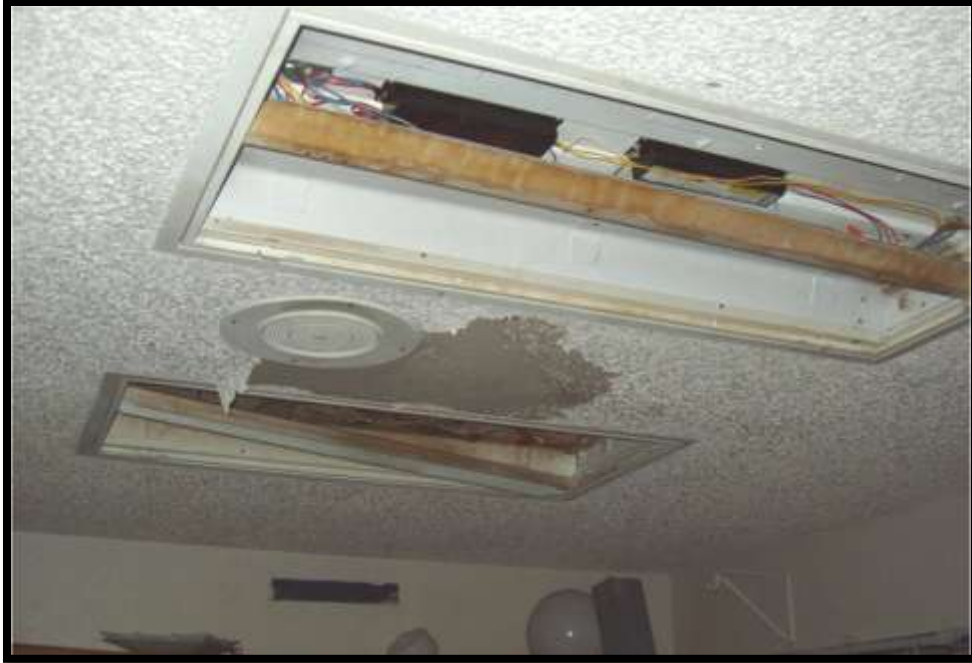
Figure 5-22. Some ceiling delamination occurred overnight.
