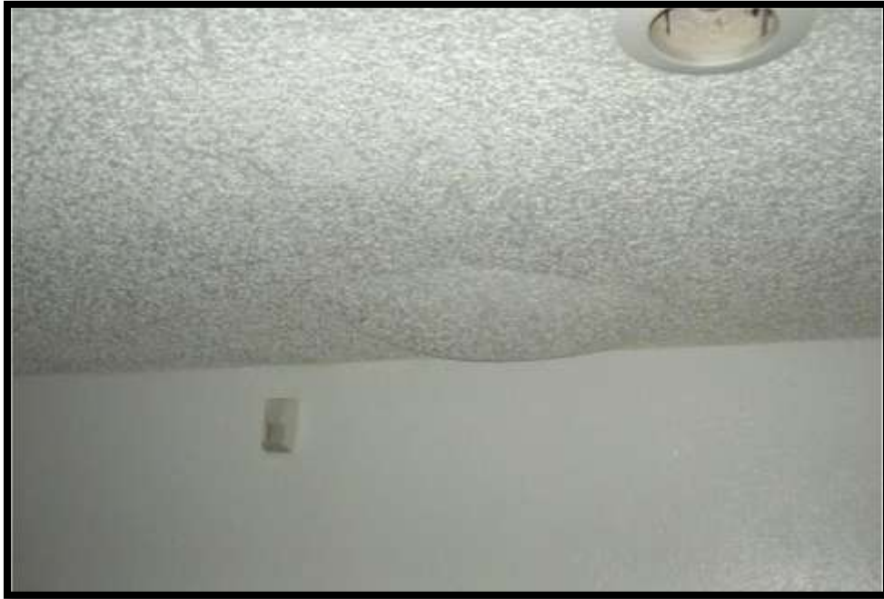
Figure 5-25. Accumulated amended water in ceiling material.
