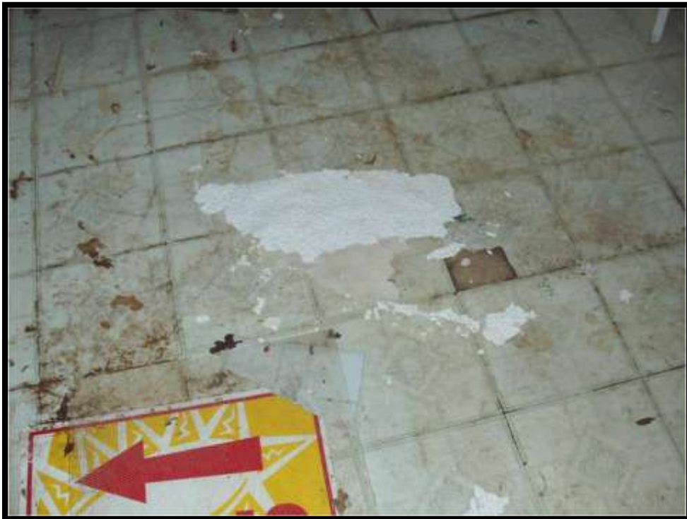
Figure 5-23. Popcorn ceiling fragments on the floor.
