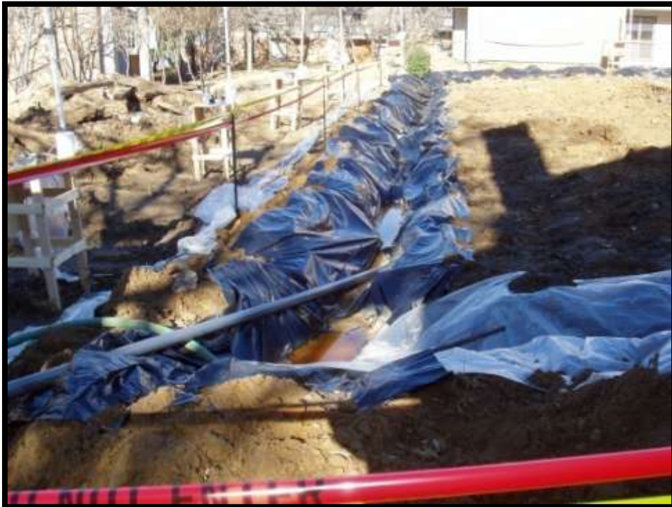
Figure 5-49. Very little water in ditch liner.
