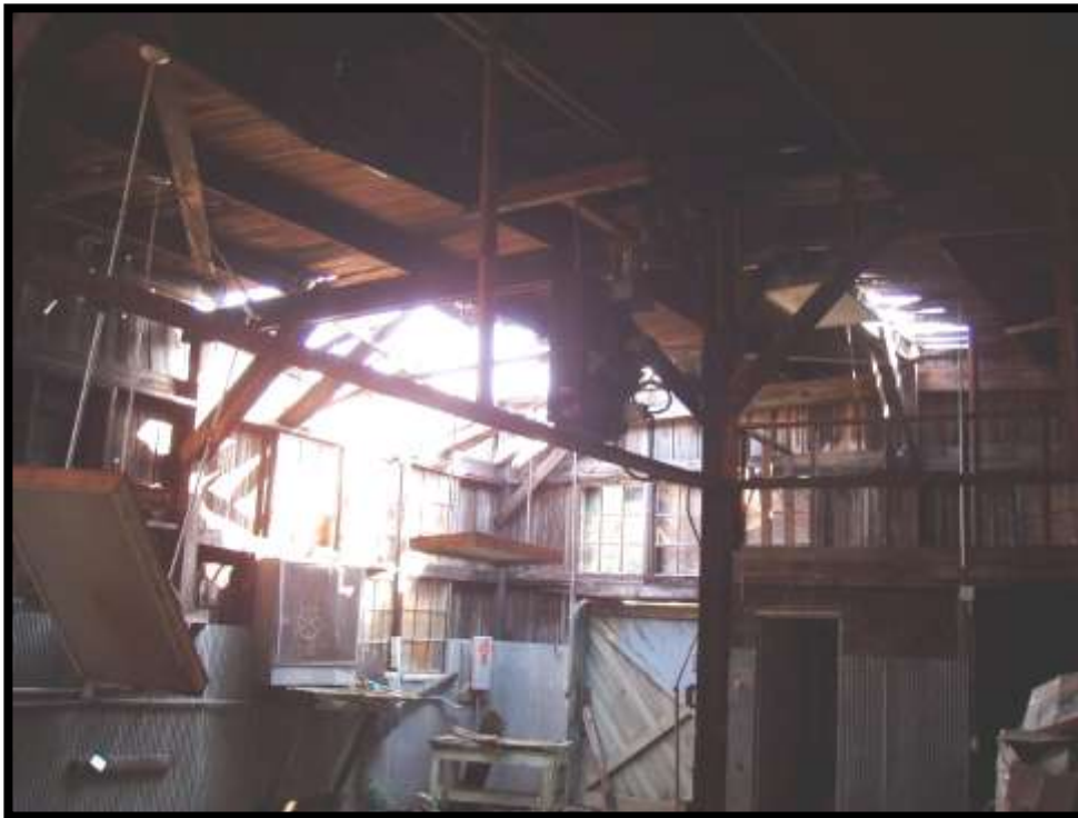
Figure 4-3. Interior view of the damaged roof in the transite building.
