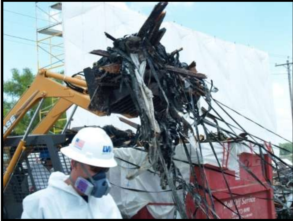
Figure 5-39. Problems caused by the Velcro stored in the building.
