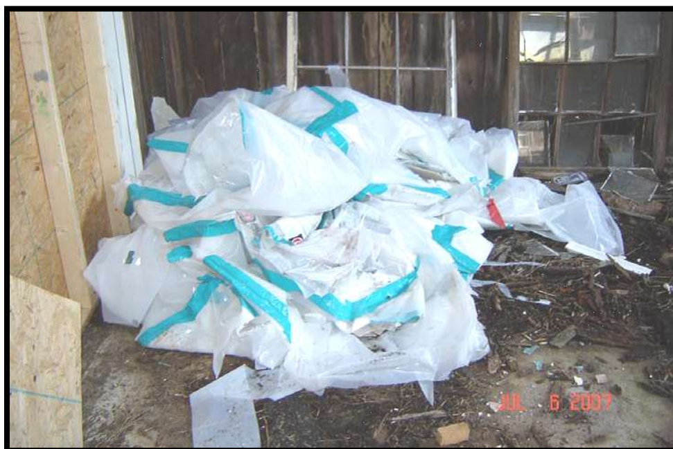
Figure 4-21. Excess transite from Fort Hood, placed in building.
