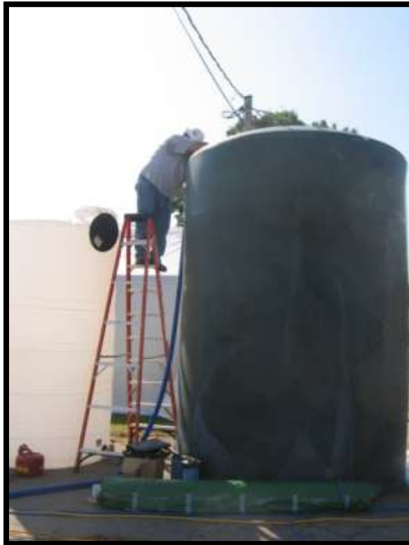
Figure 5-10. Water holding tank and filtration system.
