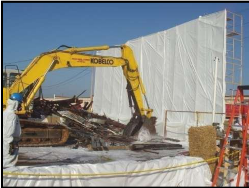
Figure 5-36. All of the transite building on the ground.
