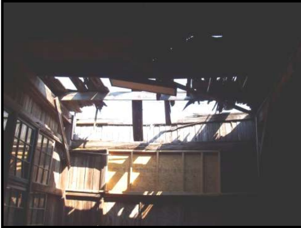
Figure 4-4. Interior view of the damaged roof in the transite building.
