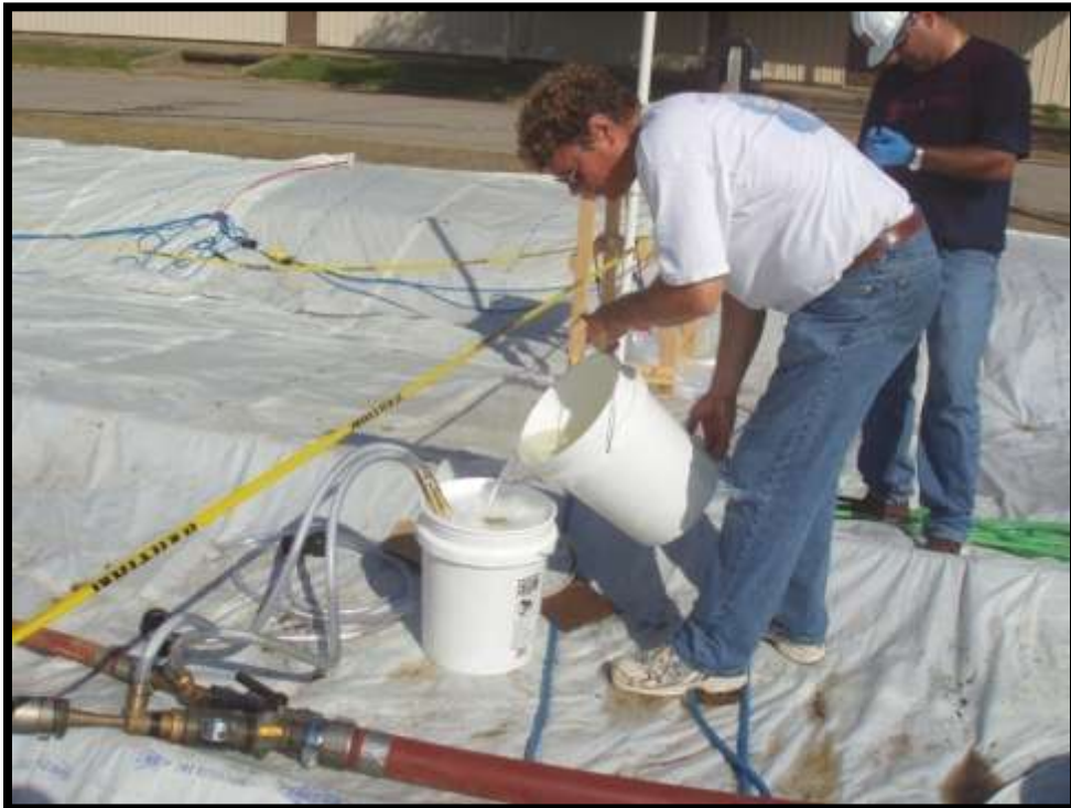
Figure 5-34. Refilling amended water supply.
