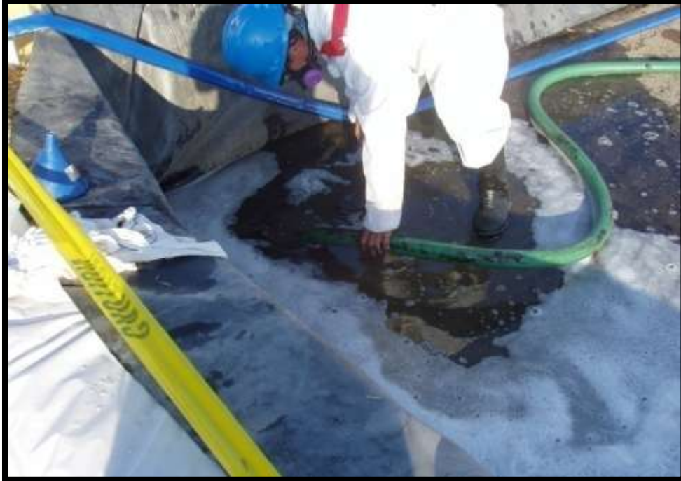
Figure 5-46. Collection sump for contaminated amended water.
