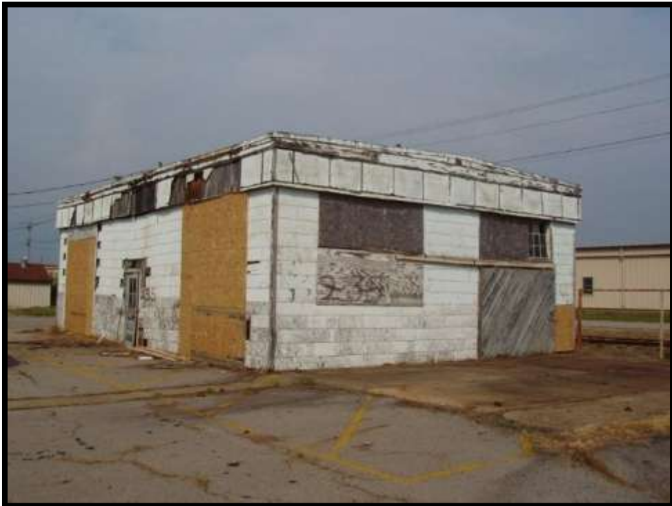
Figure 4-9. The building before the additional transite.
