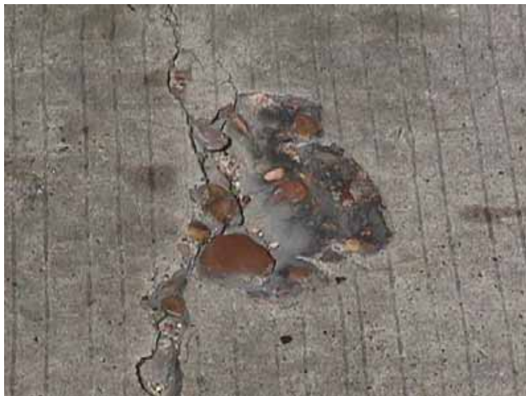
Figure 54. Round-shaped aggregates at a spalled CRCP crack.
