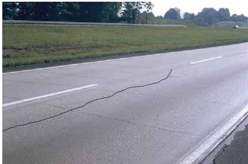
Figure 20. Longitudinal crack in CRCP due to thermal shock. Crack is enhanced for clarity.
