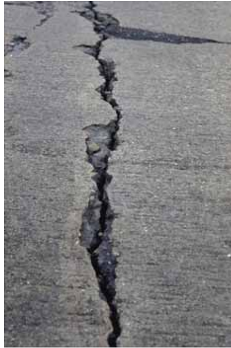
Figure 59. Photograph of deflection spalling on a CRCP.
