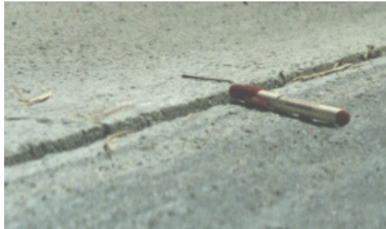
Figure 26. Photograph of faulting in JPCP.
