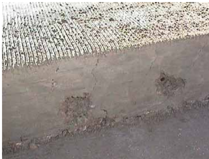
Figure 18. Plastic shrinkage cracking in concrete pavement.
