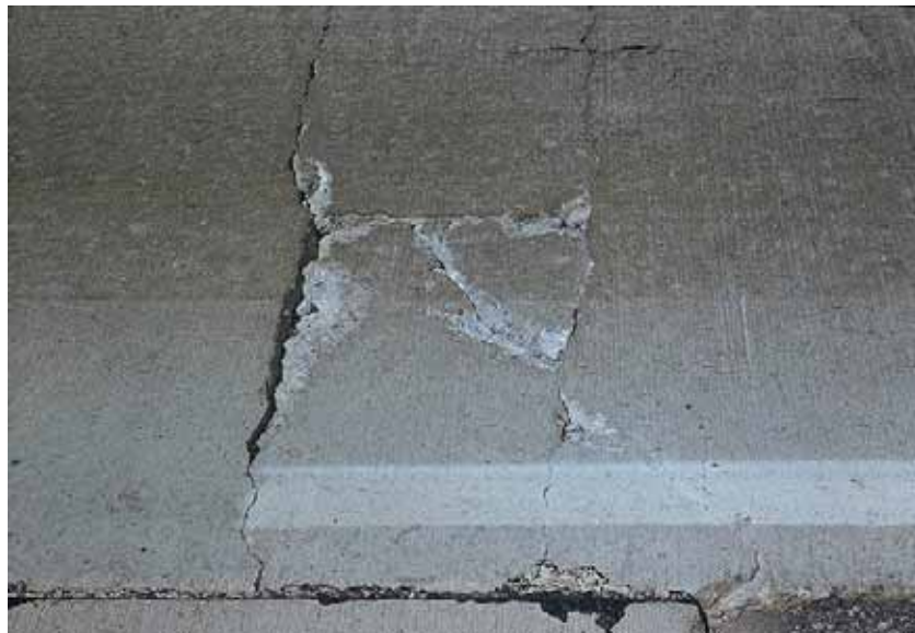
Figure 64. Typical CRCP punchout distress.
