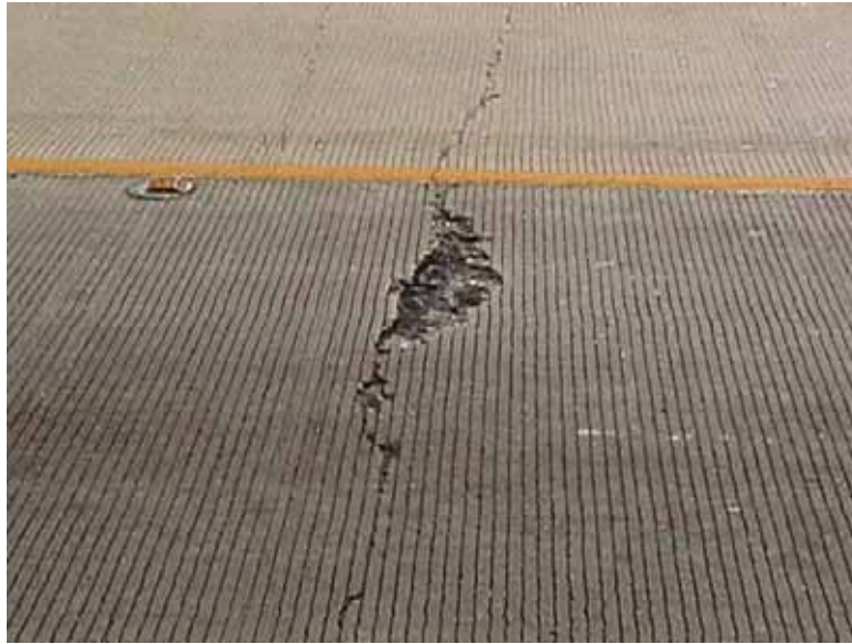
Figure 53. Delamination spalling at a CRCP crack.
