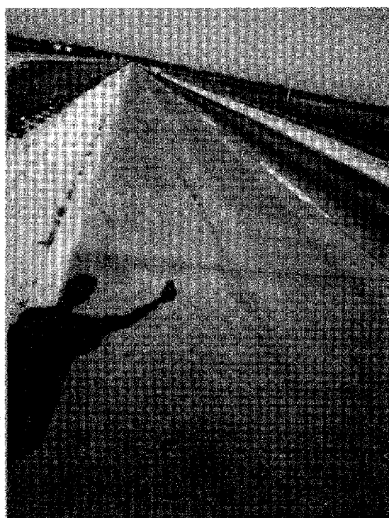
(a) Staining along longitudinal cracks
