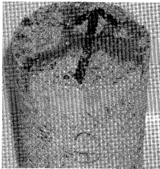
Figure 3-75. Map cracking pattern on core CA-014-011-001E, emphasized by wetting down the surface.
