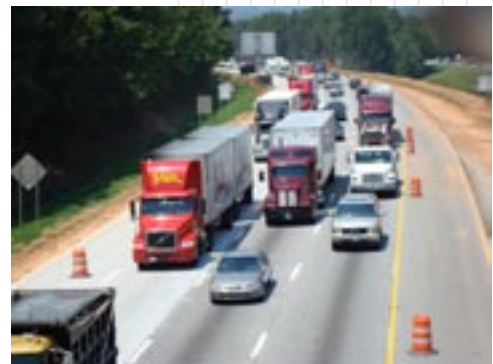
Figure 2. The I-75, Georgia, reconstruction of asphalt pavement using jointed concrete pavement during 32 weekend full closures.
