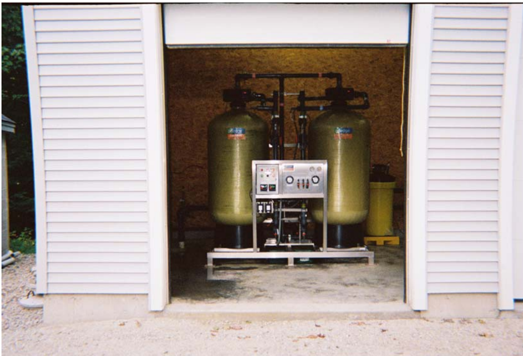
Figure 4-5. APU-100 Treatment System
