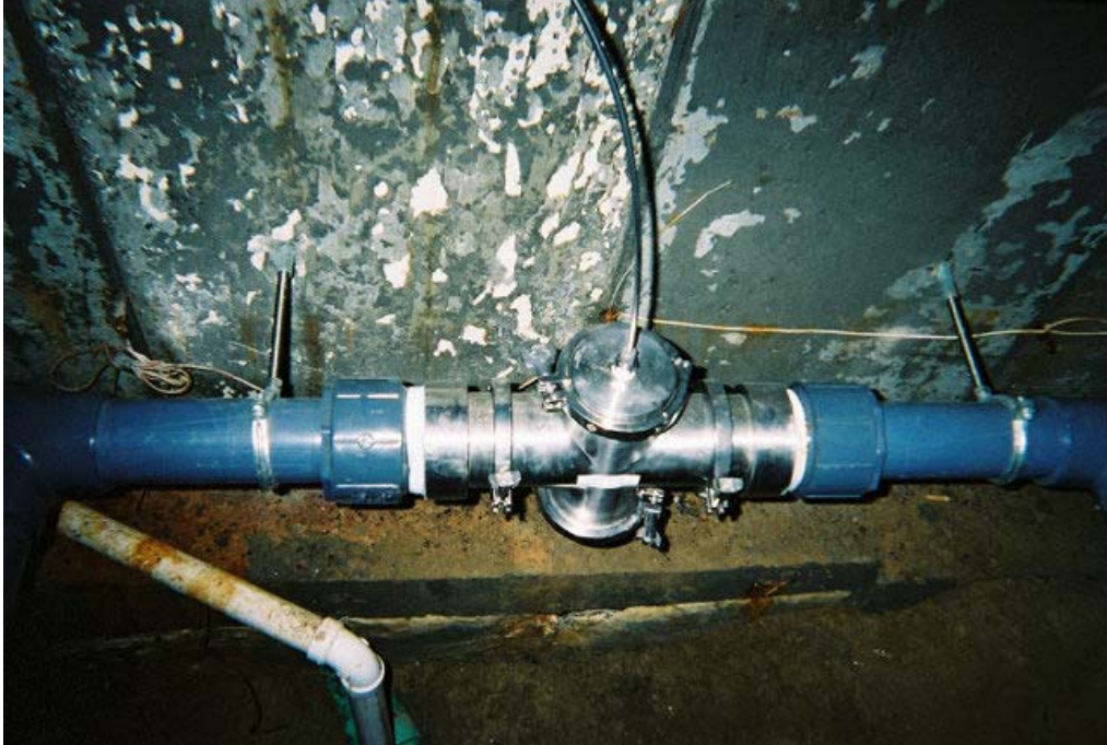
Figure 4-4. Gas Injection Point for the CO 2 System Used for pH Adjustment
