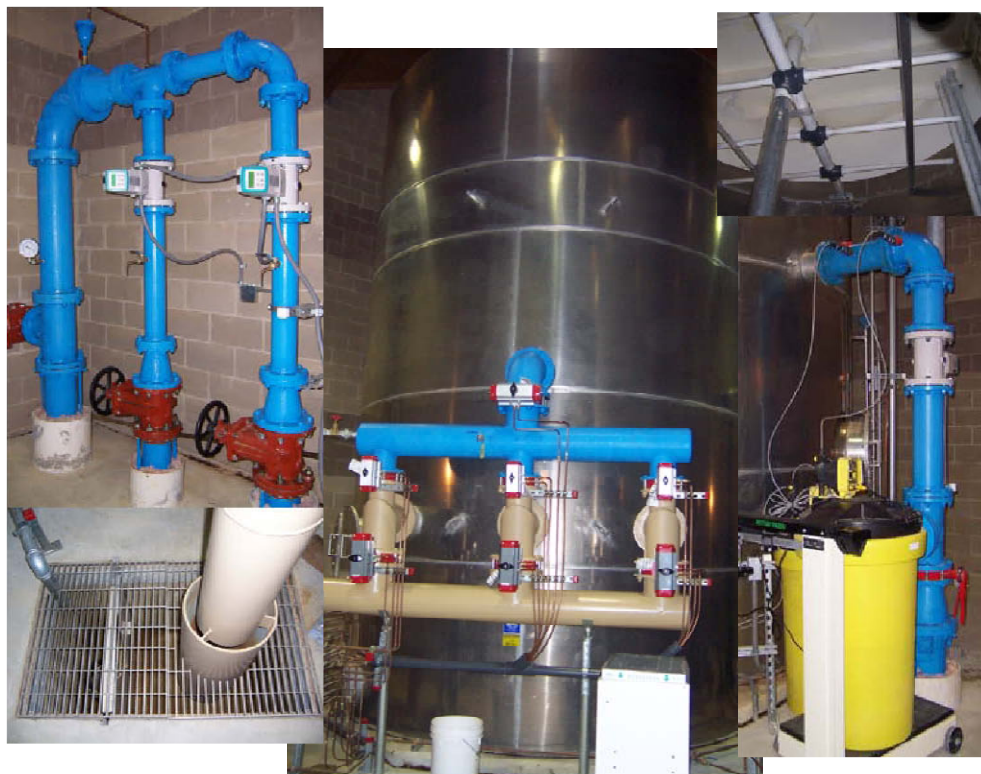
Figure 4-5. Treatment System Components
