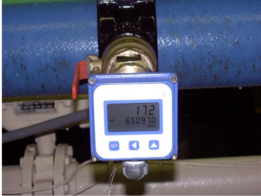
FIGURE 5-3. Filter Effluent Flow Meter
