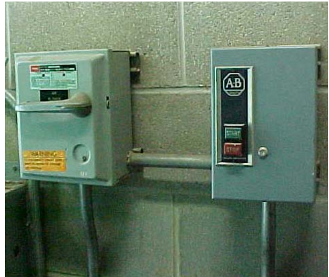
FIGURE 5-6. Air Wash Blower Controls
