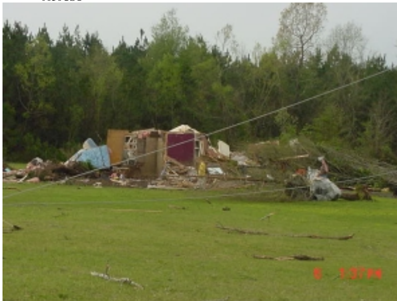
F3 damage to a home in the Monterey Community.
