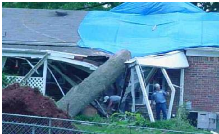
Home damaged due to tree being uprooted and falling on residence in Underwood-Petersville community. Photo taken by WCM Tim Troutman.
